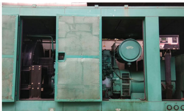
Diesel engine generator
