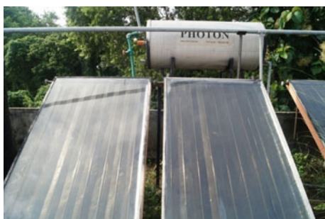
Solar water heater
